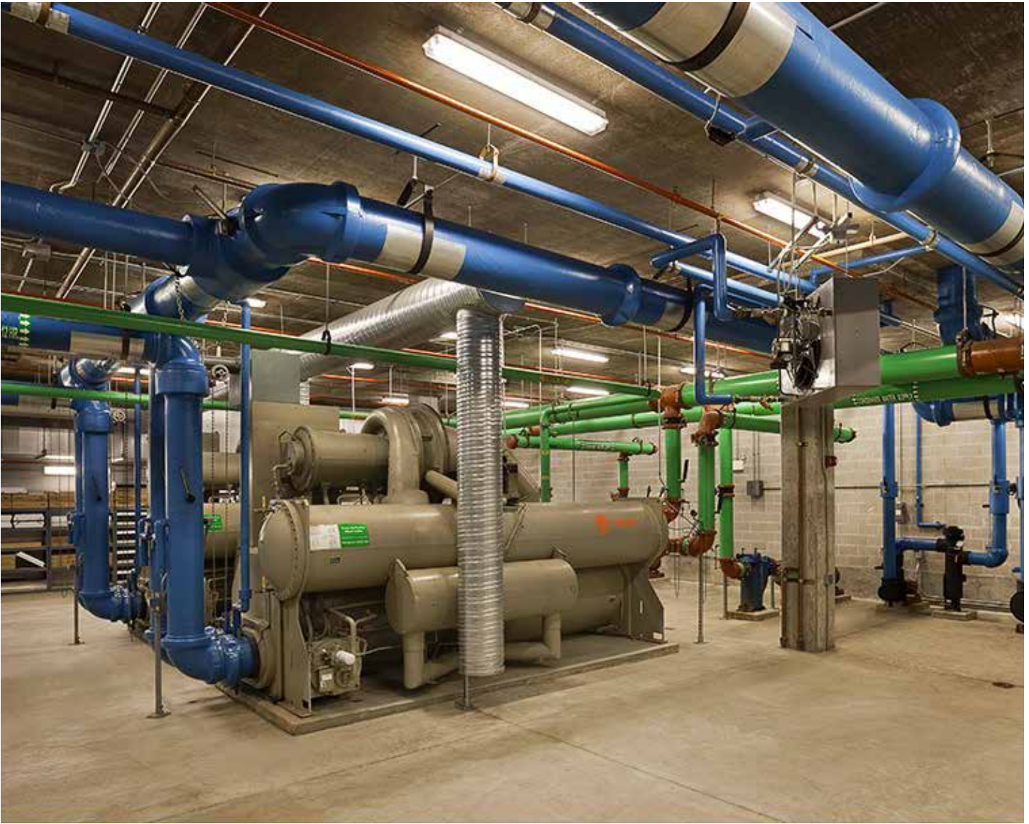
The chiller plant at the FBI Chicago Regional Office. Adjustment of the sequencing of the cooling system was one change among many that helped to bring the building's Energy Star rating to 90.
