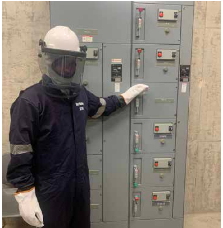
Engineer Cory Lane demonstrating arc flash gear.
