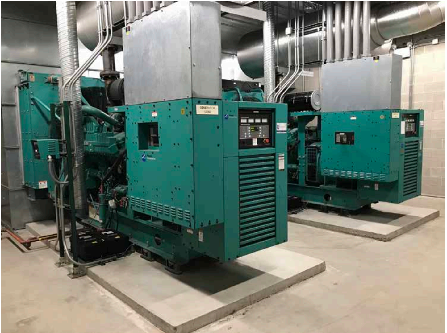
Twin emergency generators at the FBI Chicago Regional Office offer redundancy and continuity for its critical infrastructure in case of power disruption.
