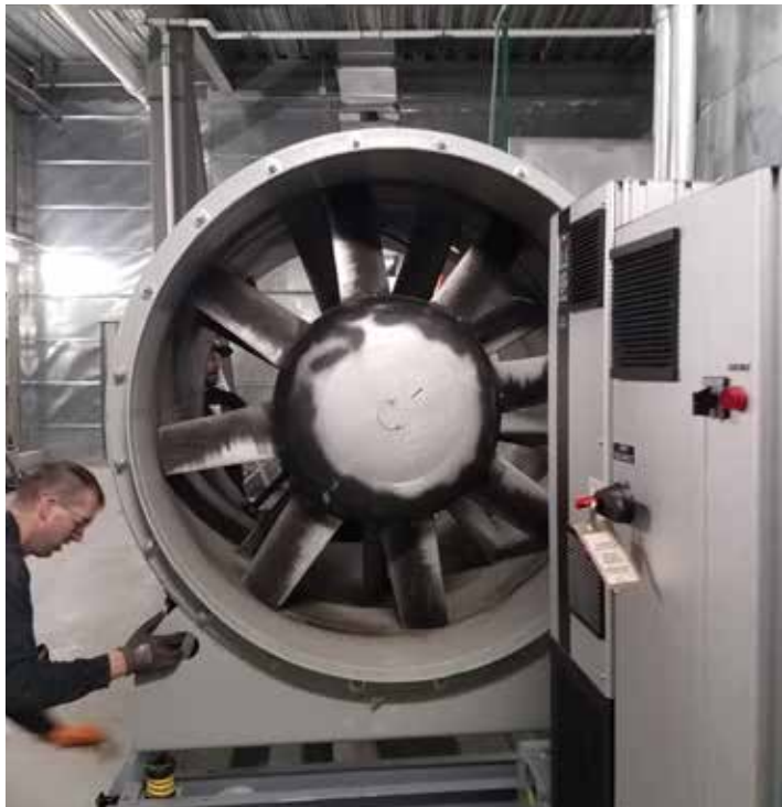
Performing a 150-horsepower motor replacement on a vane axial fan system. Planned projects include a fan wall retrofit.
