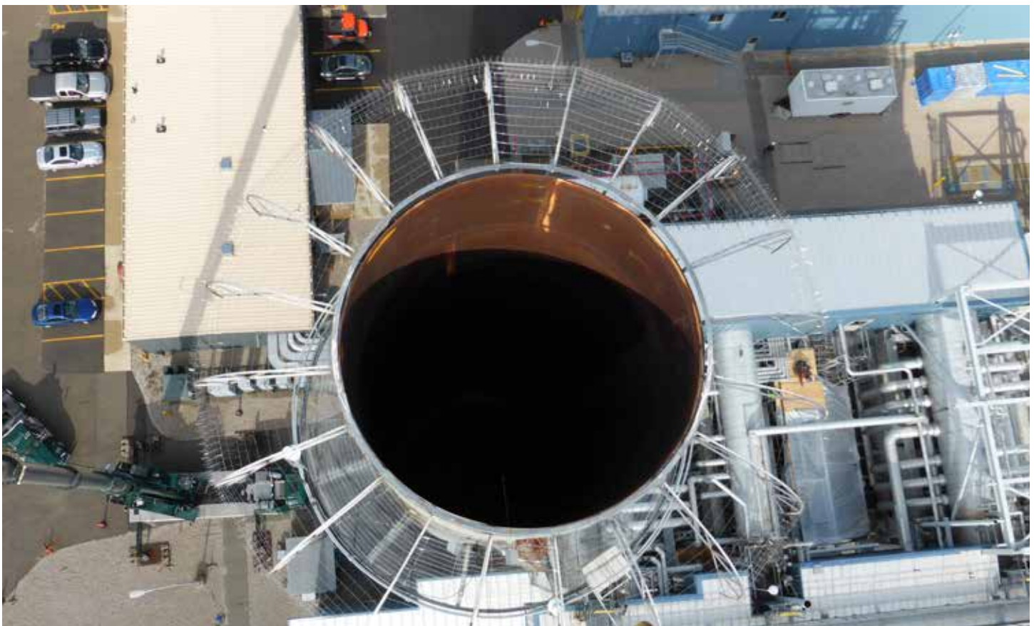
Comprehensive lightning protection measures help keep peaker plants in a constant state of readiness.
