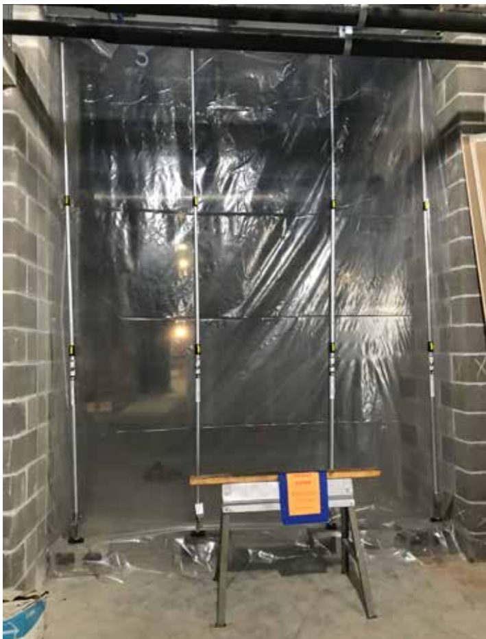
Proper inspection of facilities early on can avoid painful and needless downtime for more serious mitigation later.
