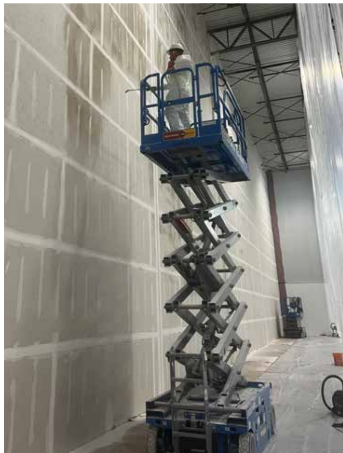
At a battery plant in Kansas City, a barrier encloses the scissor lift needed to treat the mold-contaminated surface high up on the facility’s wall.
