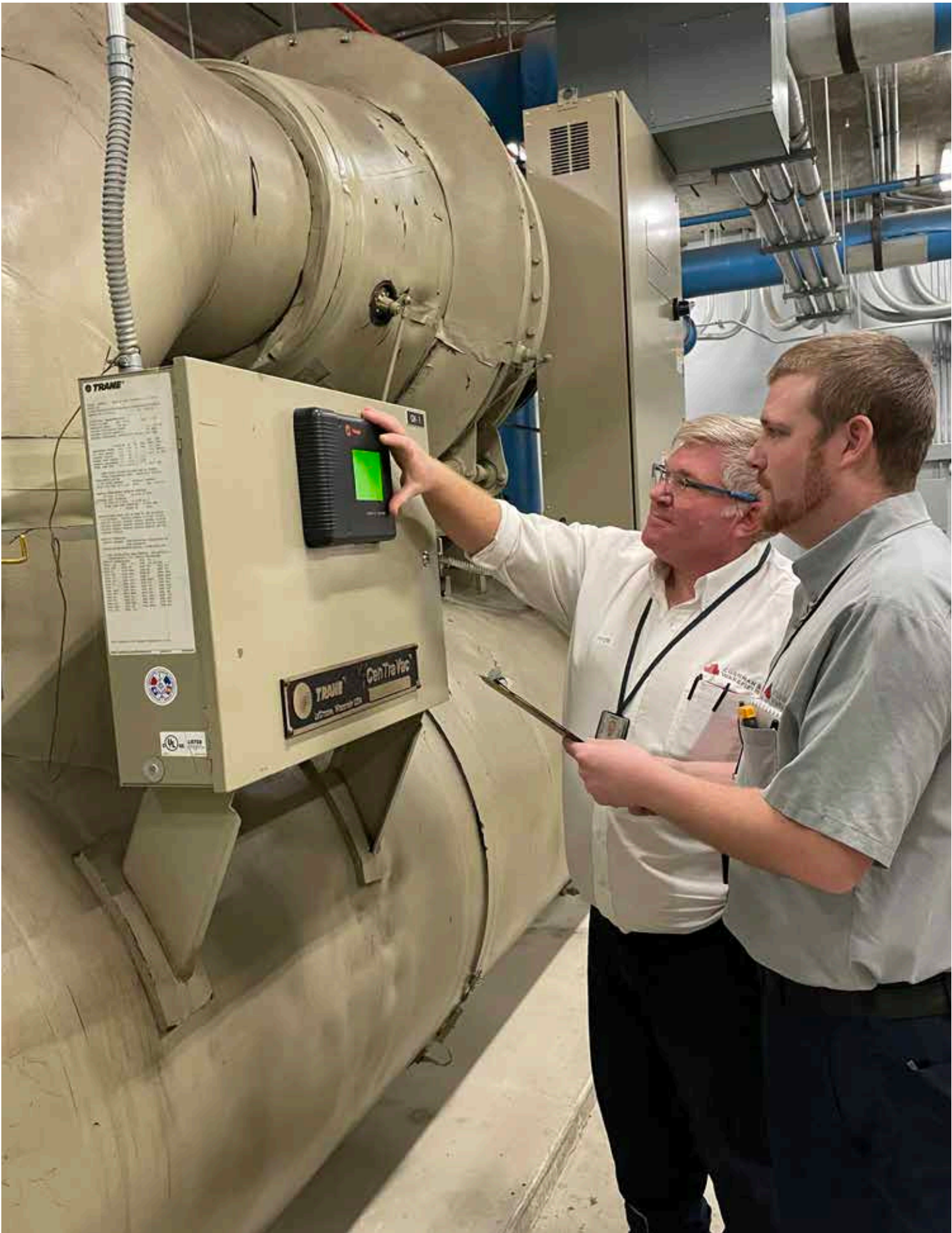
Chief Engineer Frank Gallina and Engineer Cory Lane take readings on a 650-ton Trane Centrifugal Chiller.
