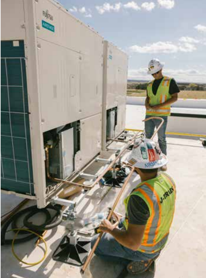
Braden Yoder and Jonathan John pipe one of several heat recovery system on the roof of the school.
