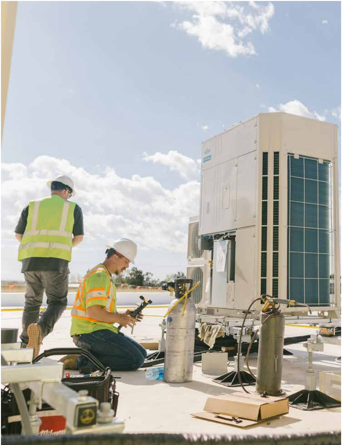
Comfort Air Mechanical technicians install Fujitsu AIRSTAGE heat recovery units on the roof of the new school.
