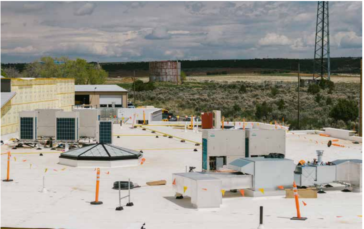
A Fujitsu AIRSTAGE VU-V heat recovery system was selected for the heating and cooling system at the new Dove Creek Elementary School.
