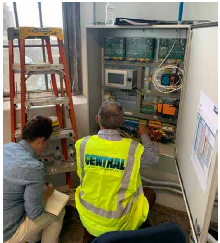
Echem Consultants provided design and installation support, with continued monitoring and maintenance, of a corrosion mitigation system, referred to as Impressed Current Cathodic Protection (ICCP), at the Tribune Tower Residences.
