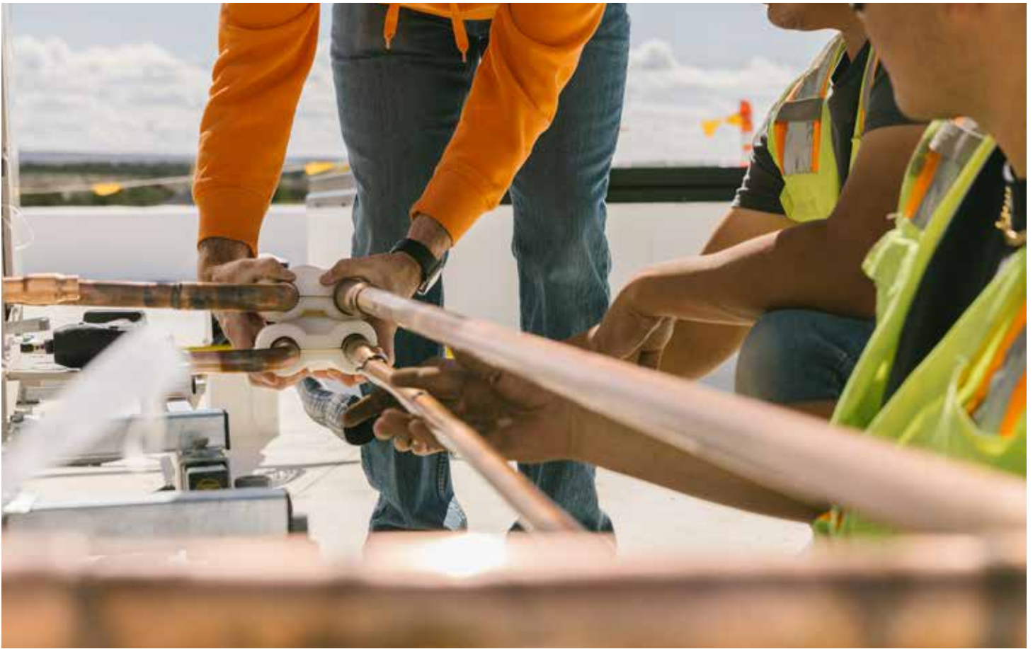
One benefit of the Fujitsu AIRSTAGE VU-V system is the ability to field-configure the system for either heat recovery or heat pump with piping changes.
