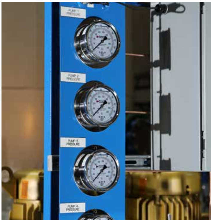
Large, easy-to-read pressure gauges take any guesswork out of monitoring of each of the four pumps in the system. (Photo: Shedd Aquarium)
