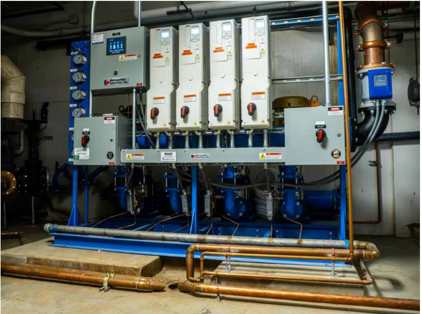
Metropolitan Industries' four-pump system fully integrated and operational at the Shedd Aquarium. (Photo: Shedd Aquarium)
