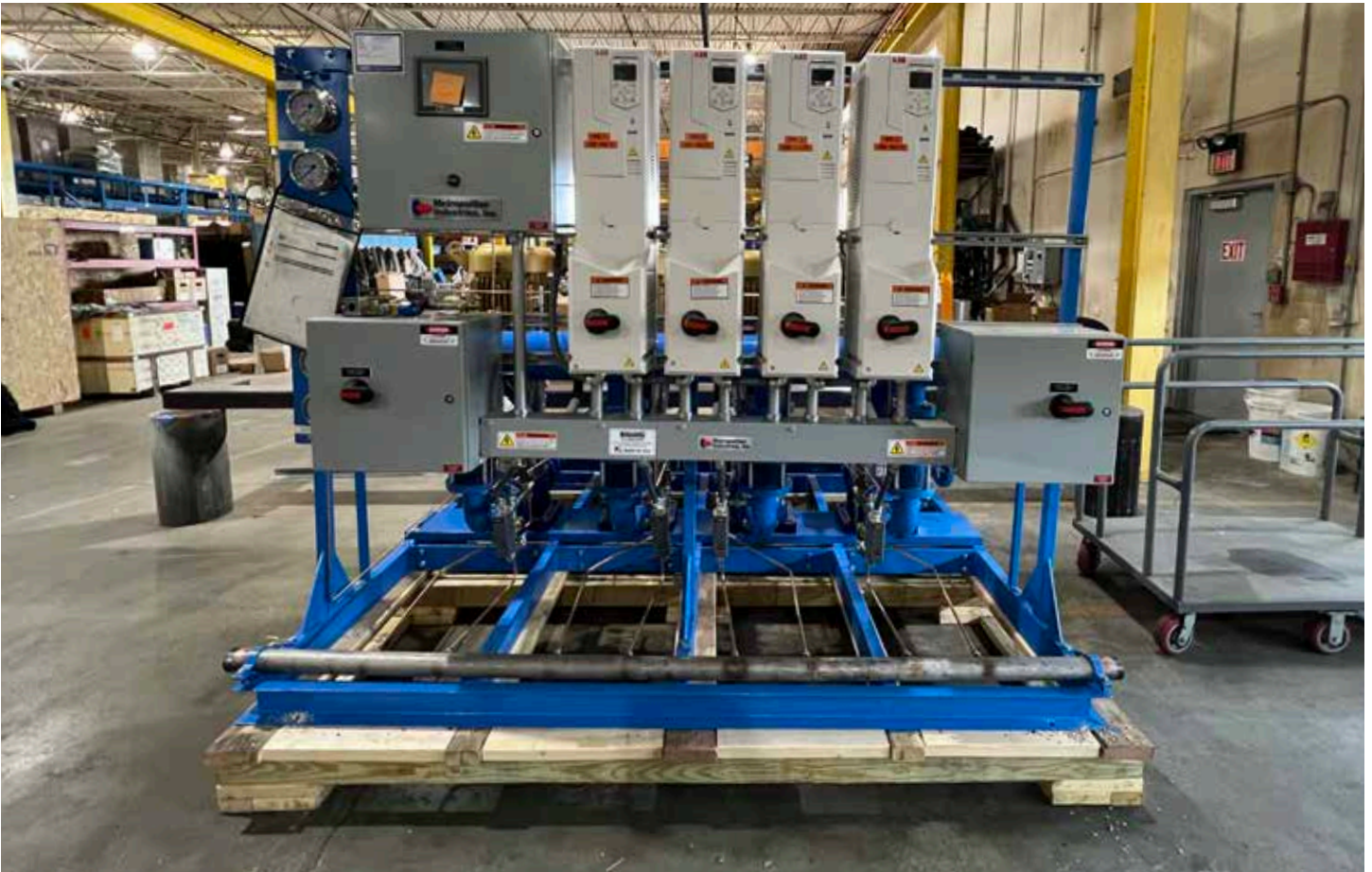
Redundancy is key to the Shedd's risk management strategy. Upgrading to a four-pump, skid-mounted system from a three-pump arrangement augments backup capacity in case one of the other pumps fails, reducing the risk of system downtime. (Photo: Shedd Aquarium)
