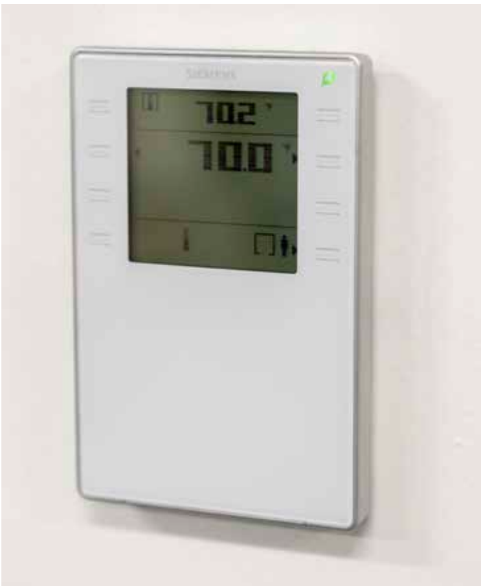
New HVAC controls in place.
