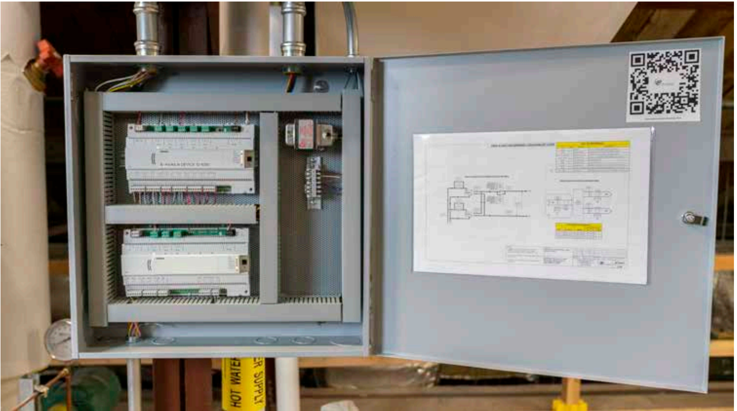
Significant benefits of IP-based controllers are their reduced upload time and ability to be programmed more efficiently.
