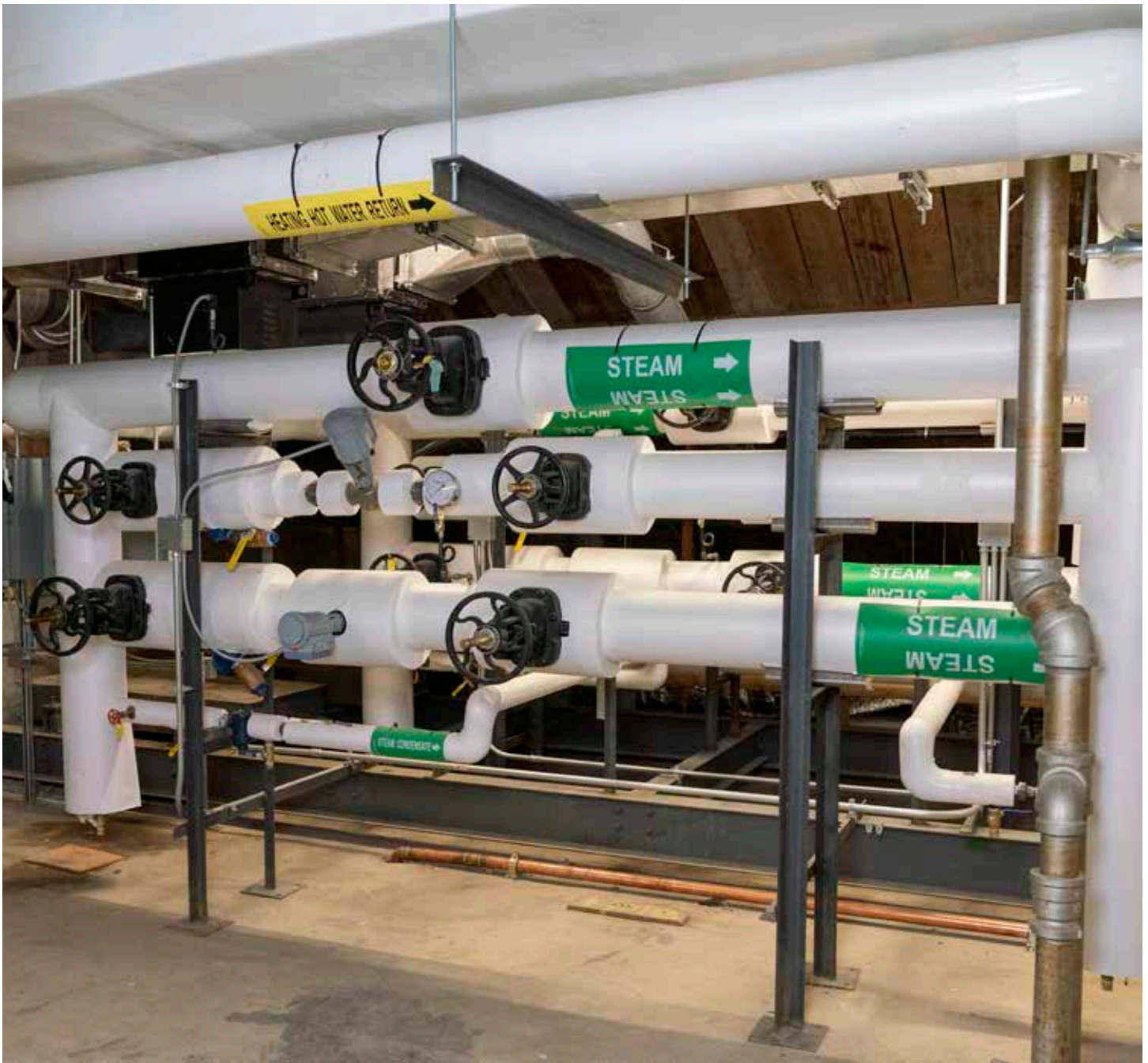
Sensors are essential to regulate equipment, to ensure comfort levels within a building and to provide chief engineers with essential data.
