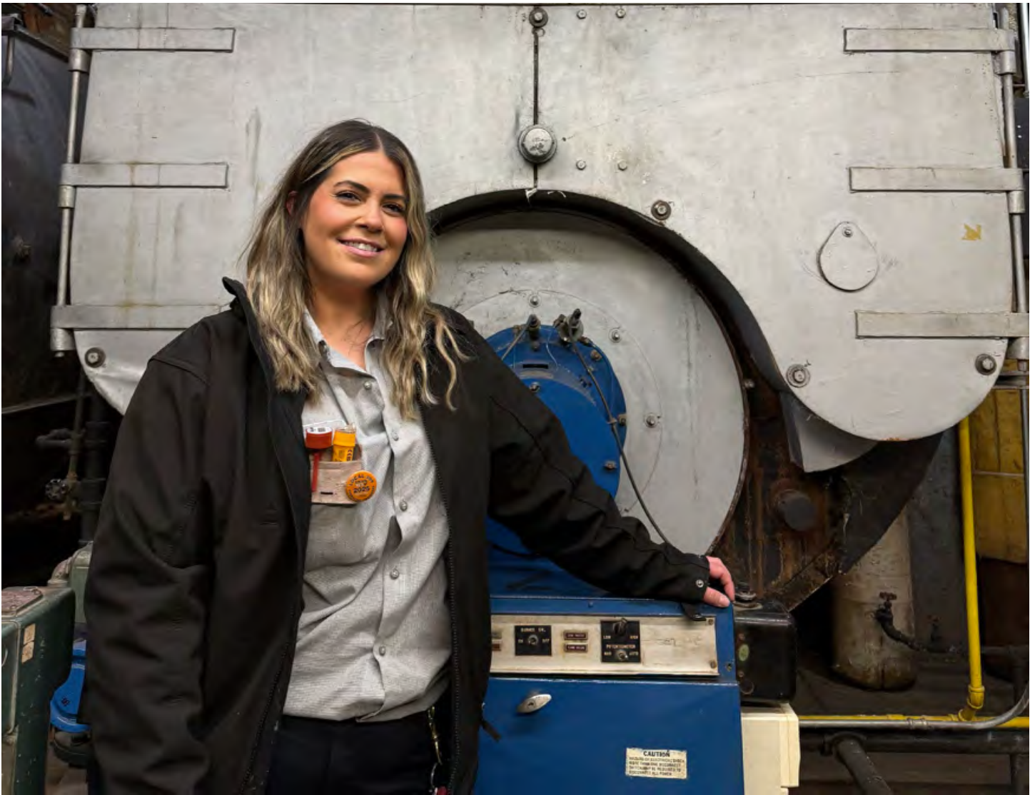
Alaniz learns by facing the same challenges that her more experienced colleagues face, from equipment like the building's boilers like the one here, to wide-ranging tenant demands, and changing expectations for the building's energy performance.
