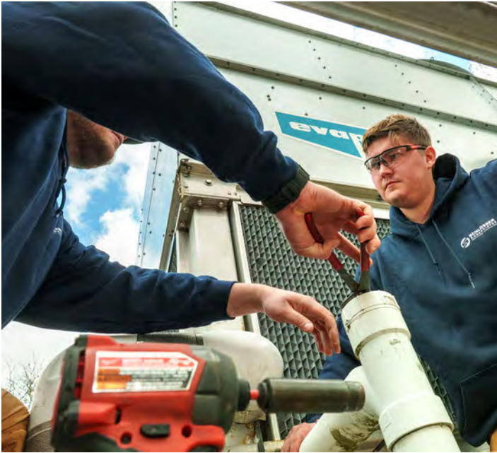
A complex network of domestic and process water piping serves the many facilities at the Siemens site.
