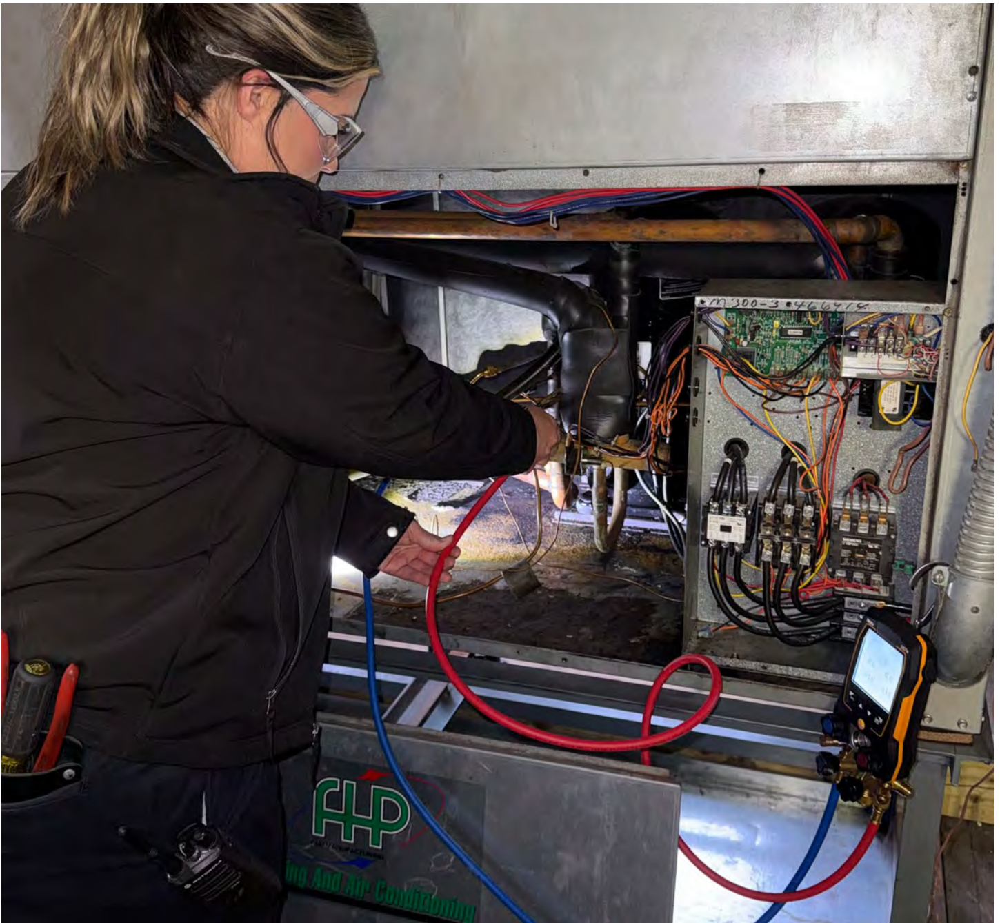
Troubleshooting a refrigeration system — part of the hands-on routine helping to make Sarah Alaniz a master of her trade.
