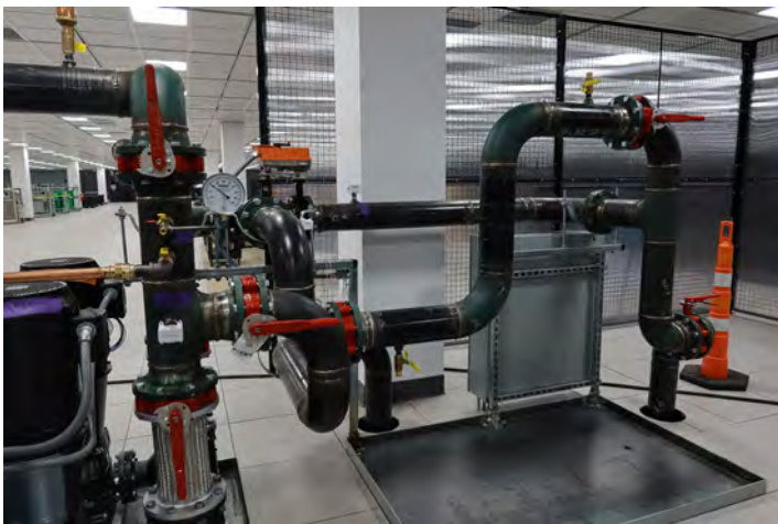
When a client needed to push chilled water through the racks at their data center Atomic Mechanical Services' team devised a solution involving a storage tank and an N+1 redundant pumping system that led to the client asking them to reproduce the results at their data centers nationwide.
