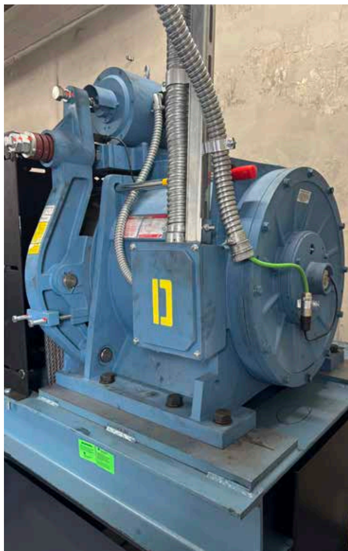
Recently installed Imperial AC gearless machine.
