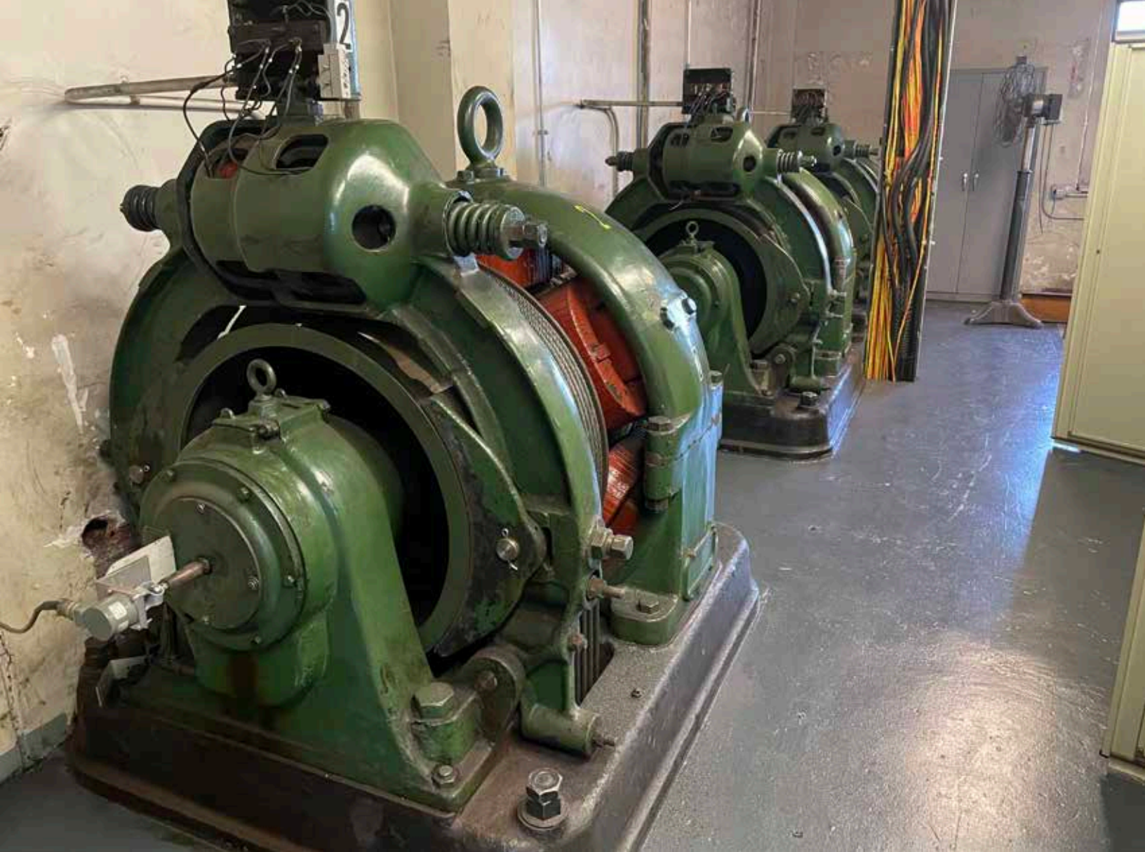
50-year-old Otis DC gearless machines.
