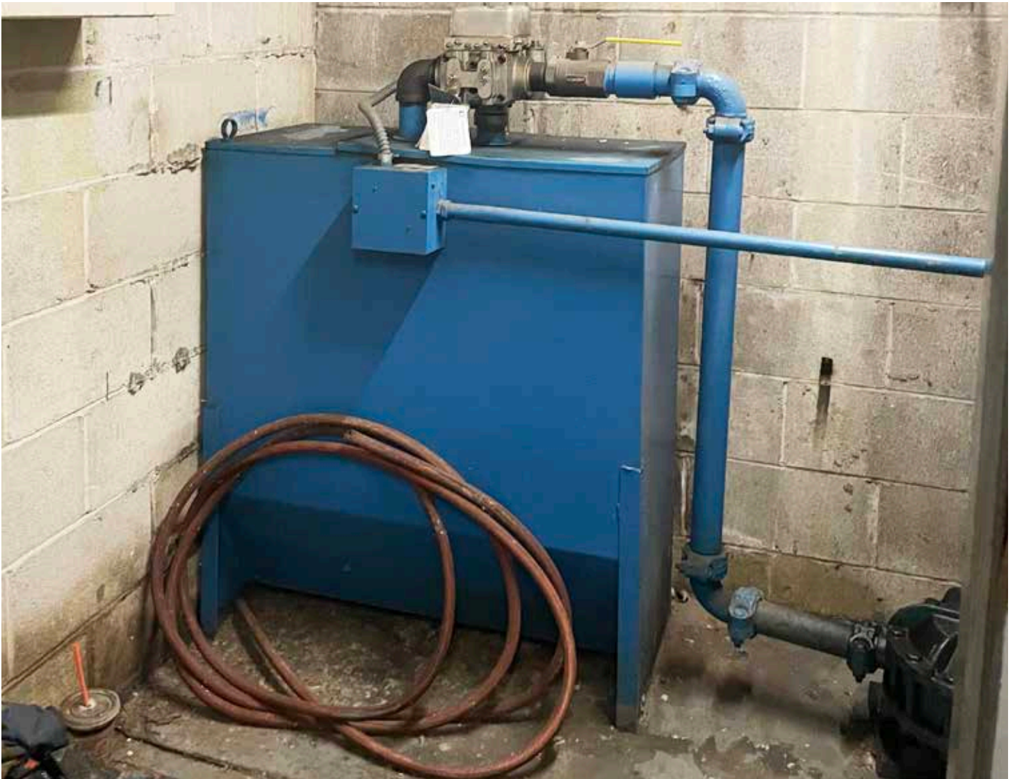
25-year-old submersible pump unit.
