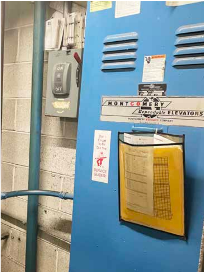
Old Montgomery hydraulic controller.
