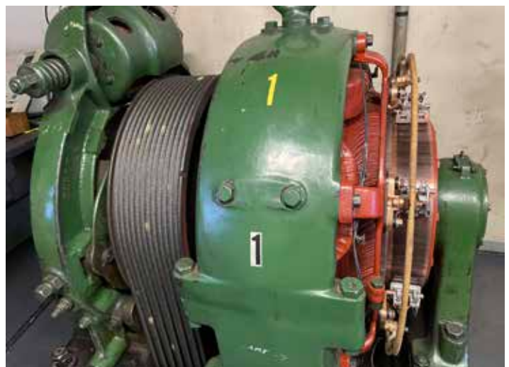
Closeup view of the Otis DC gearless machine.
