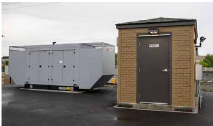
The storm water station and control building, prefabricated at the Metropolitan Industries facility in Romeoville, ready for delivery and installation in Munster, Ind.
