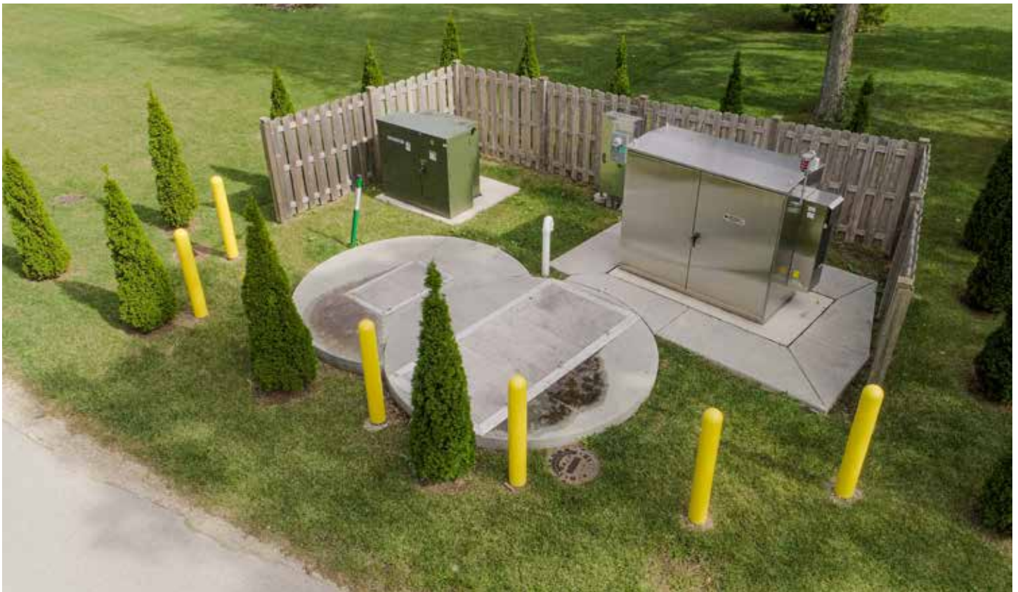
The below-ground storm water pump station in Prospect Heights' Arlington Countryside suburb is sizable enough to accommodate 2,244 gallons per minute, but effectively blends in with its surroundings.
