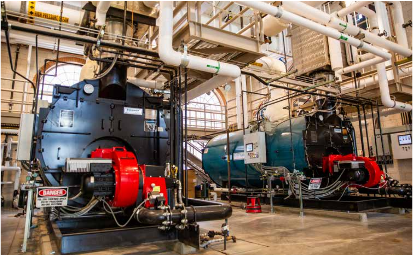
Two of the three 6,700 MBH, four-pass firetube Burnham commercial steam boilers. Jutting from the boilers, in front, are large red Weishaupt oil-fired burners. (Photo: Burnham Photos by Natalie Bee)
