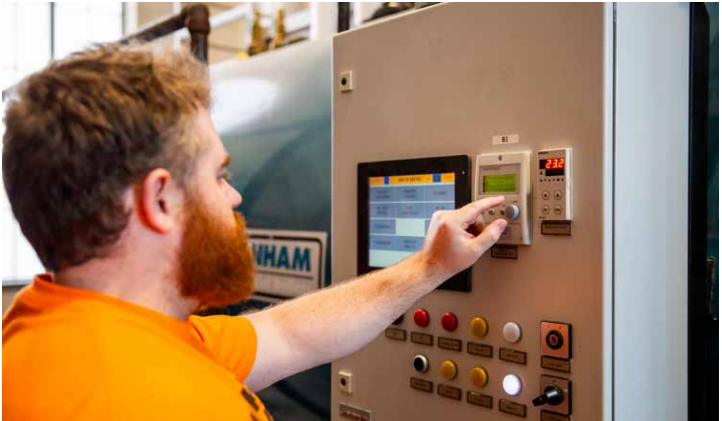
Flow between the surge tank and the deaerator are determined by the DA's feedwater level, ultimately helping to maintain optimal system performance. (Photo: Burnham Photos by Natalie Bee)
