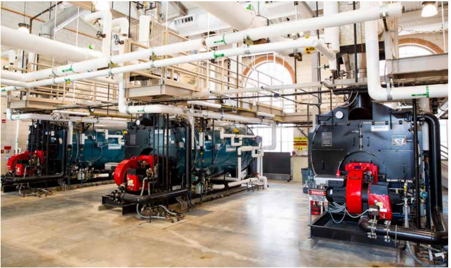
All three of the Burnham Commercial steam boilers are connected in a lead-lag configuration. Combined, the boilers provide greater capacity than is required, allowing for full redundancy of operation. (Photo: Burnham Photos by Natalie Bee)
