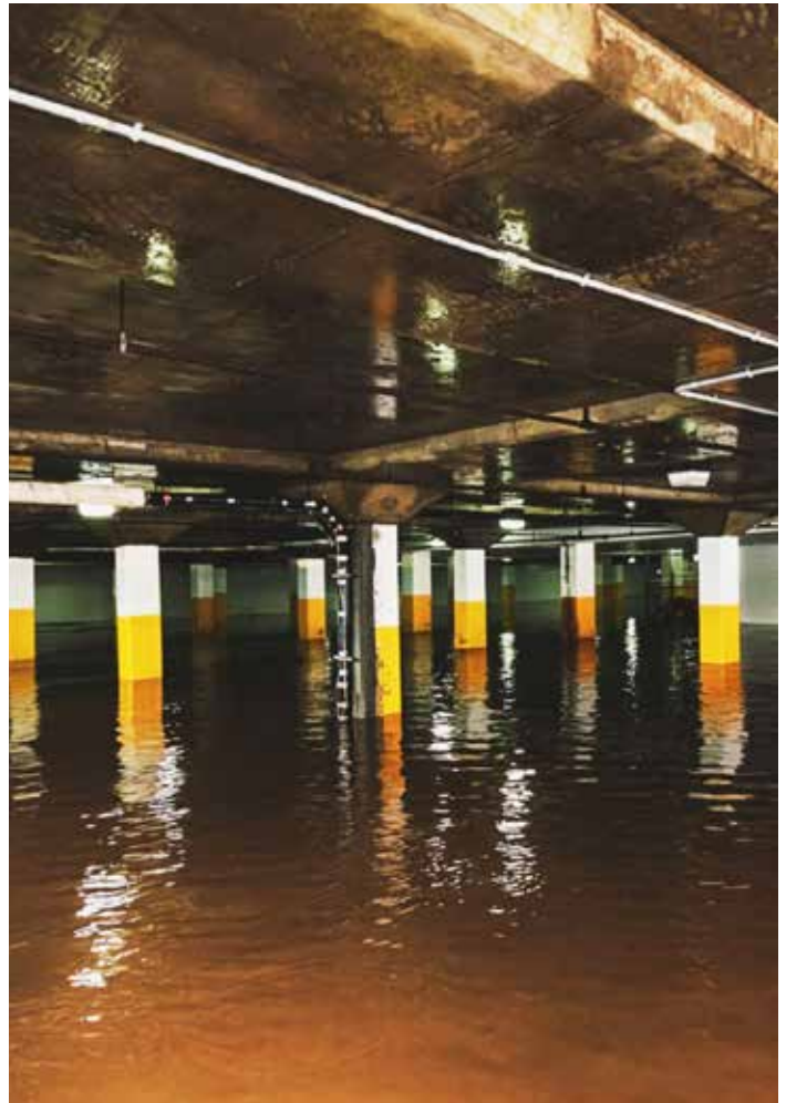
Having an evacuation plan in place prior to any onsite flooding can help you to avoid confusion, prevent injuries and limit property damage.
