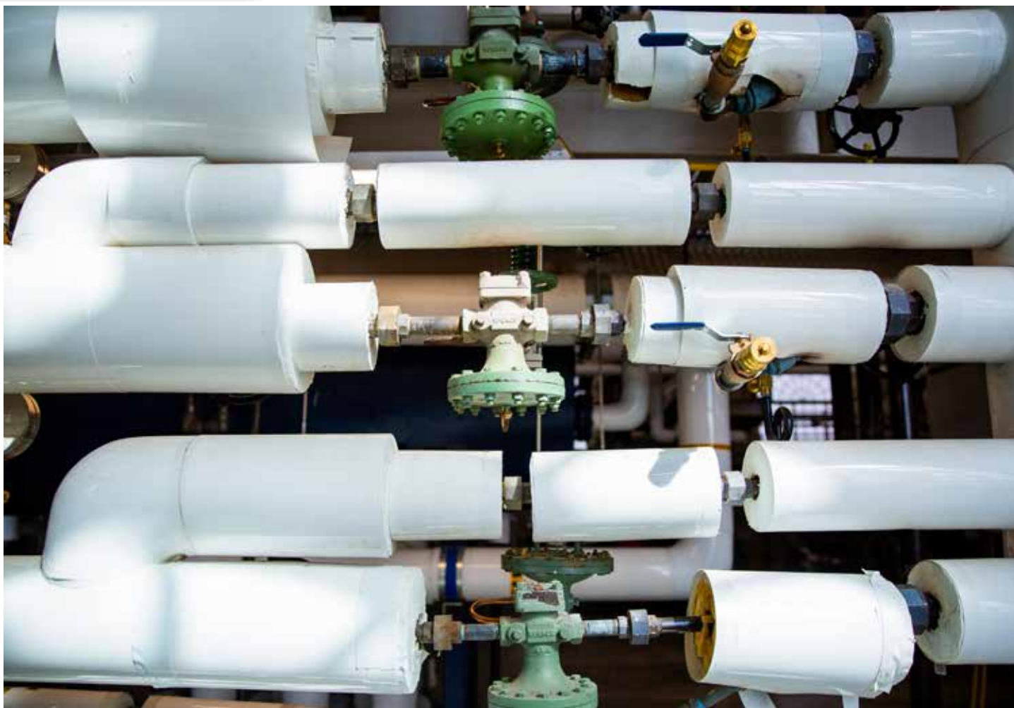
Insulated steam piping at Eastern State Hospital. (Photo: Burnham Photos by Natalie Bee)
