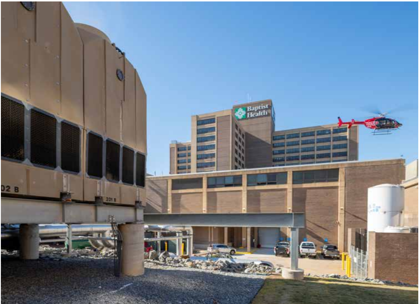
This century-old facility's decision to replace its aging wooden cooling tower gave way to a comprehensive mechanical system overhaul aimed at significantly reducing energy consumption.
