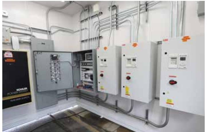
The control building inside the Evergreen Park lift station — all components made in-house at Metropolitan Industries, along with the structure itself.
