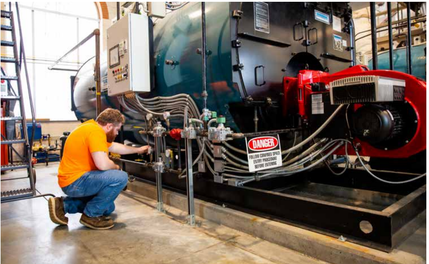
A technician performs routine maintenance to one of the three large Burnham Commercial steam boilers at Eastern State Hospital. (Photo: Burnham Photos by Natalie Bee)
