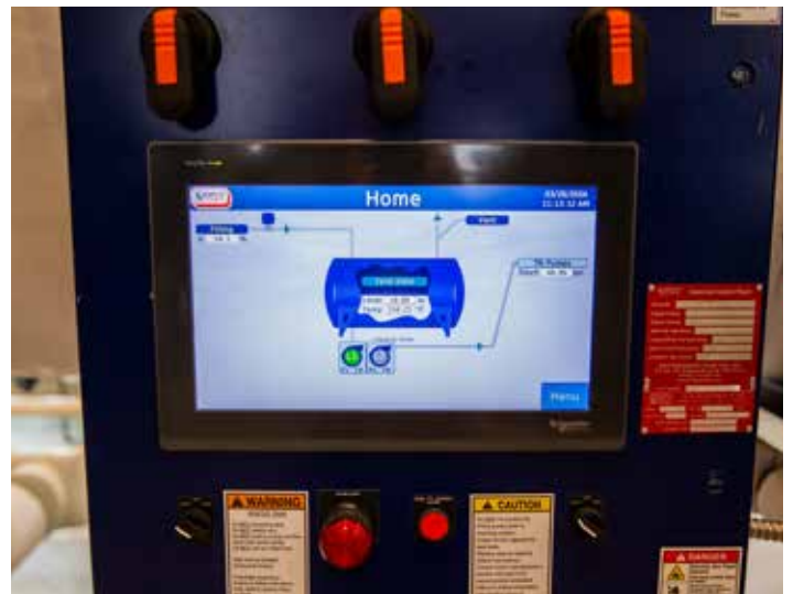
Modernizing the facility's infrastructure was an absolute priority for this retrofit. (Photo: Burnham Photos by Natalie Bee)
