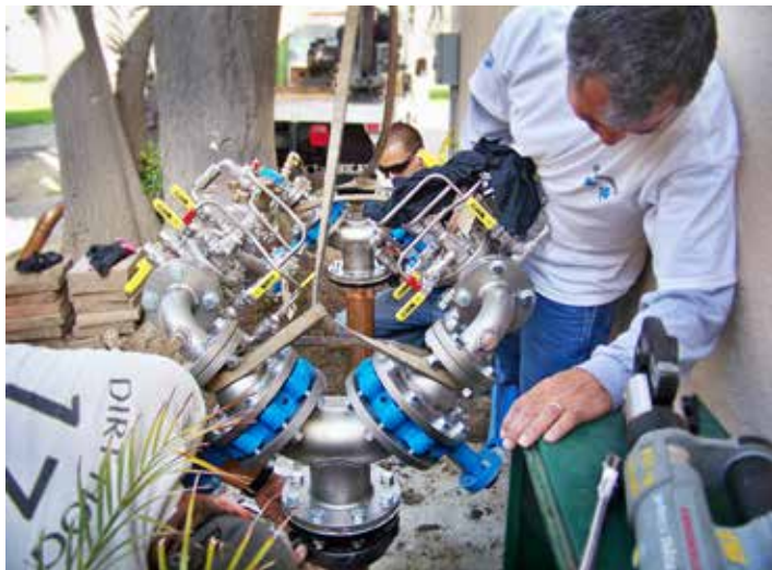
When there's no risk of freezing temperatures, new backflow assemblies are typically installed outdoors, often protected by fencing and/or locked containers.
