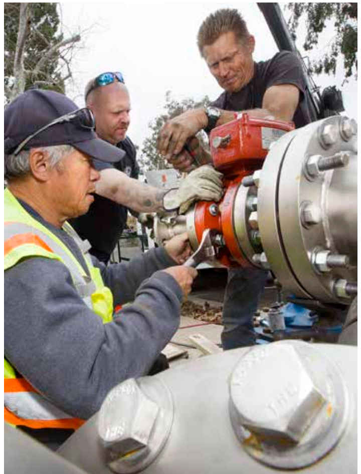
Preassembly of components, above ground, for a large backflow assembly, to be fully constructed in a bunker underground.
