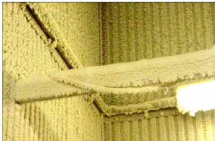
Combustible dust accumulated on overhead structural components historically has been associated with cascading secondary explosions that lead to major or total facility loss.
