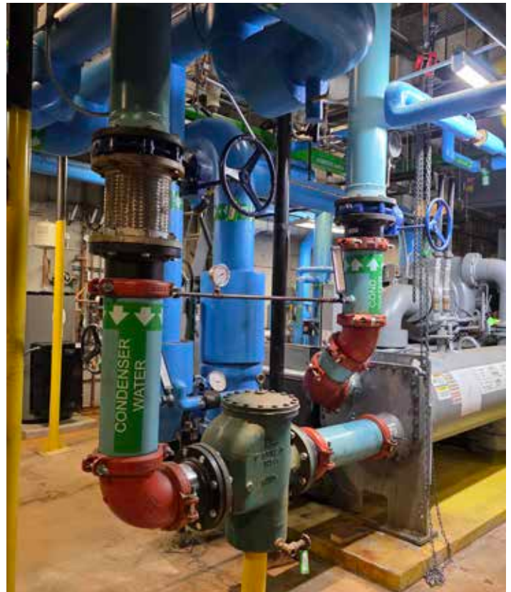
The Adler Planetarium’s main chiller plant.
