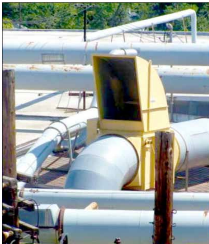
Buildings with known combustible dust hazards should be equipped with relief vents or abort gates to direct damaging pressure or burning material out of confined areas.
