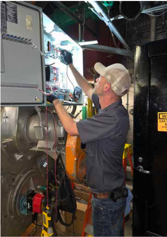
Michael Coffman installs a Cleaver-Brooks Hawkeye control system for the no. 1 250 hp boiler.
