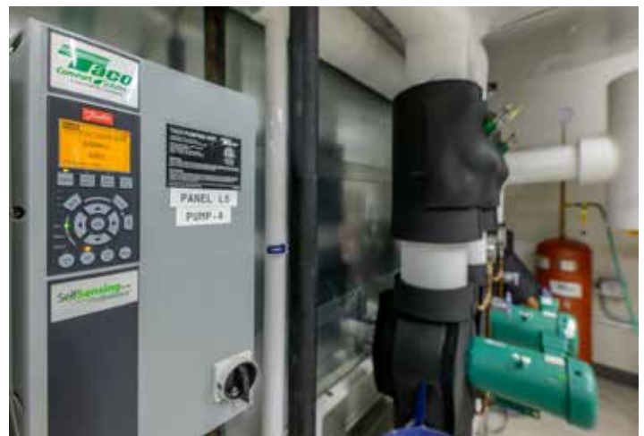
The VFDs that serve the Taco SKV pumps are manufactured by Danfoss.
