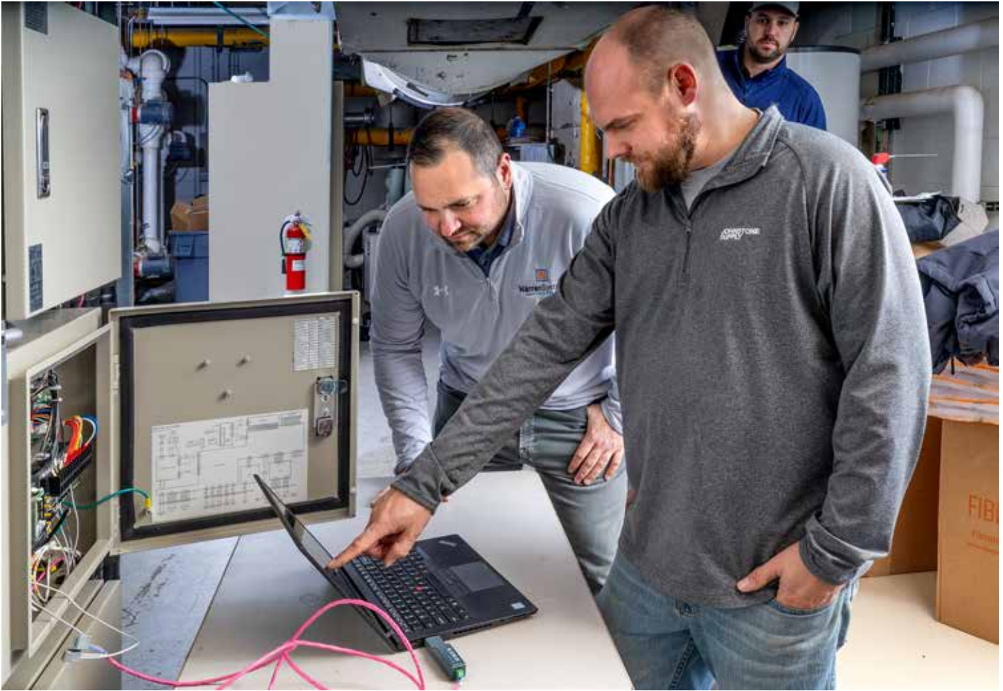
Johnstone Supply's Skylar Kaczanowski reads VRF system sensors with Ben and Landon Warren.
