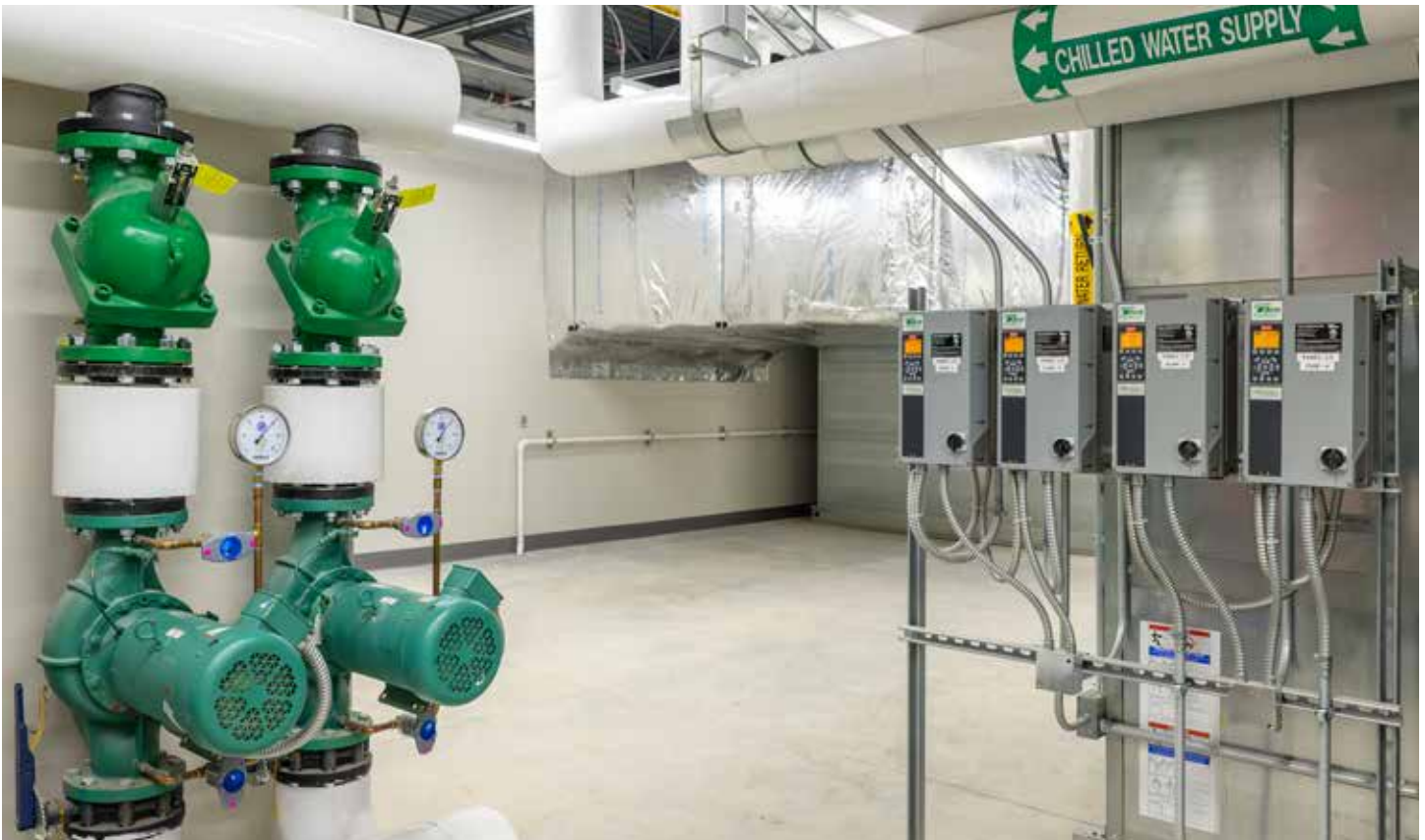
On the left, two of the Taco SelfSensing SKV pumps are shown; the VFDs (variable frequency drives) are mounted to the right.
