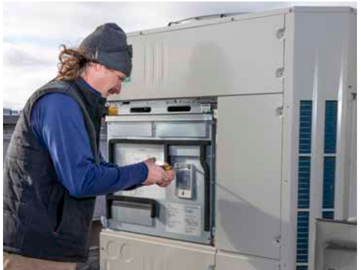
Service technician Troy Lawson accesses the VU-V control panel.
