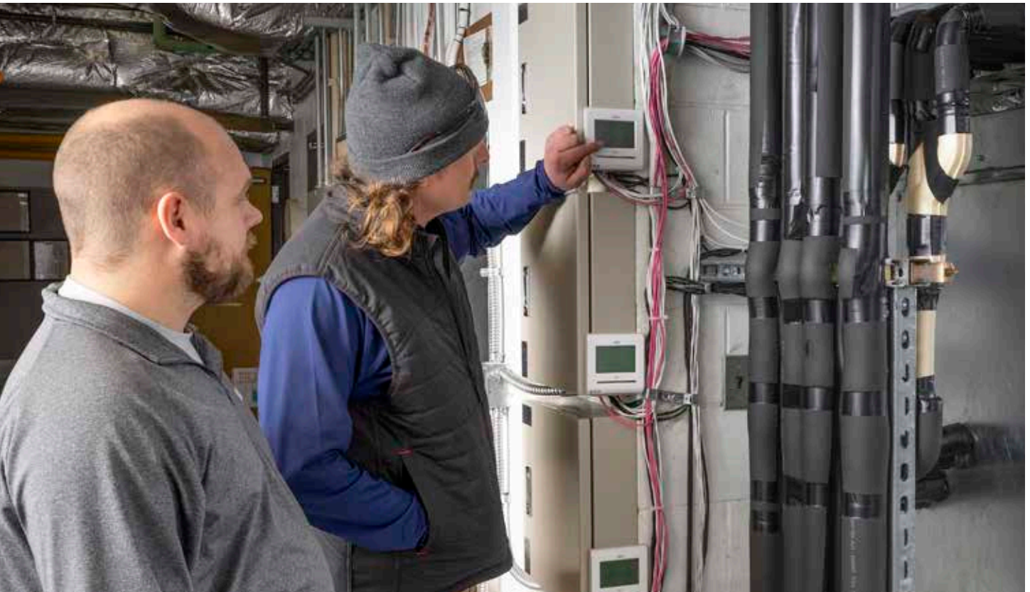
Ben Warren and service technician Troy Lawson discuss system thermostats in the mechanical room.
