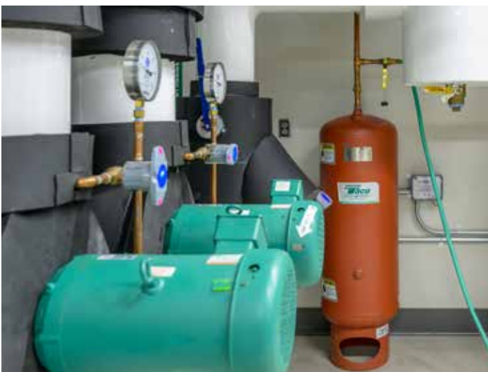
Key components of the mechanical system include Taco SelfSensing pumps, and a Taco buffer tank.
