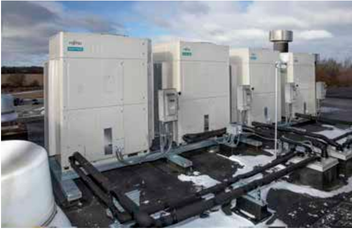
Four 10-ton Fujitsu VU-V systems were installed to supply cooling and supplementary heat to the medical facility.
