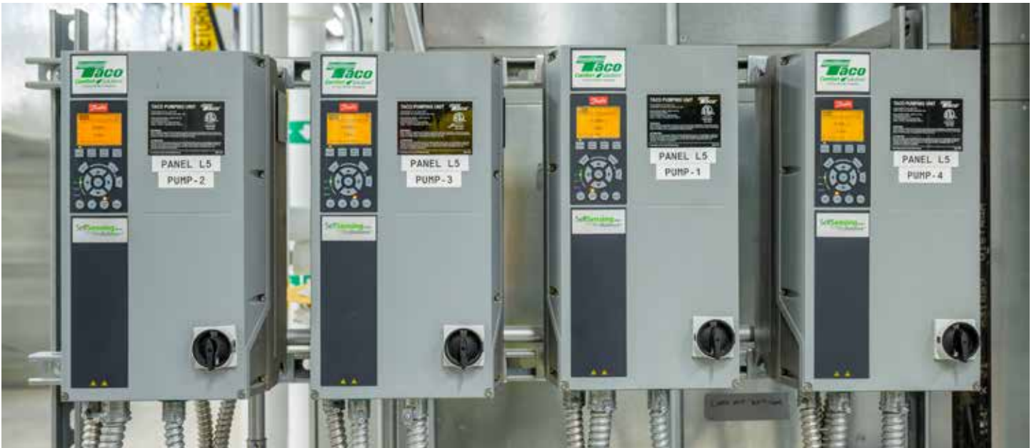
VFDs, shown here, are connected to the Taco SelfSensing SKV pumps.
