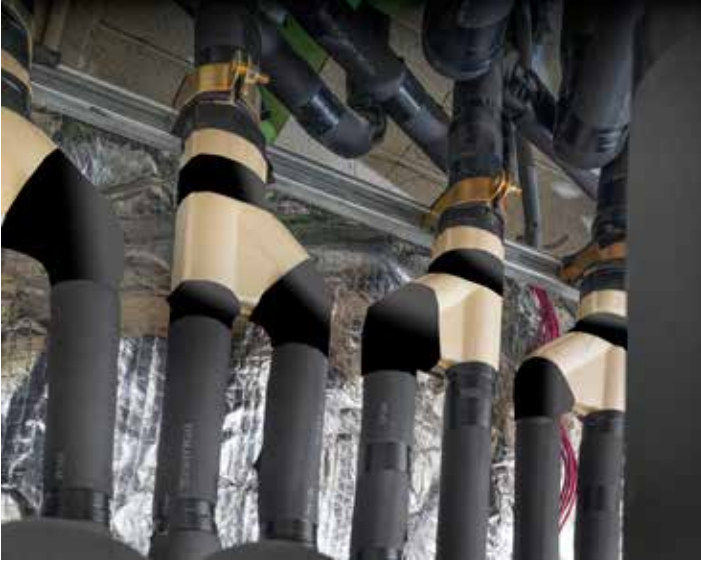
Insulated expansion valves in the mechanical room.
