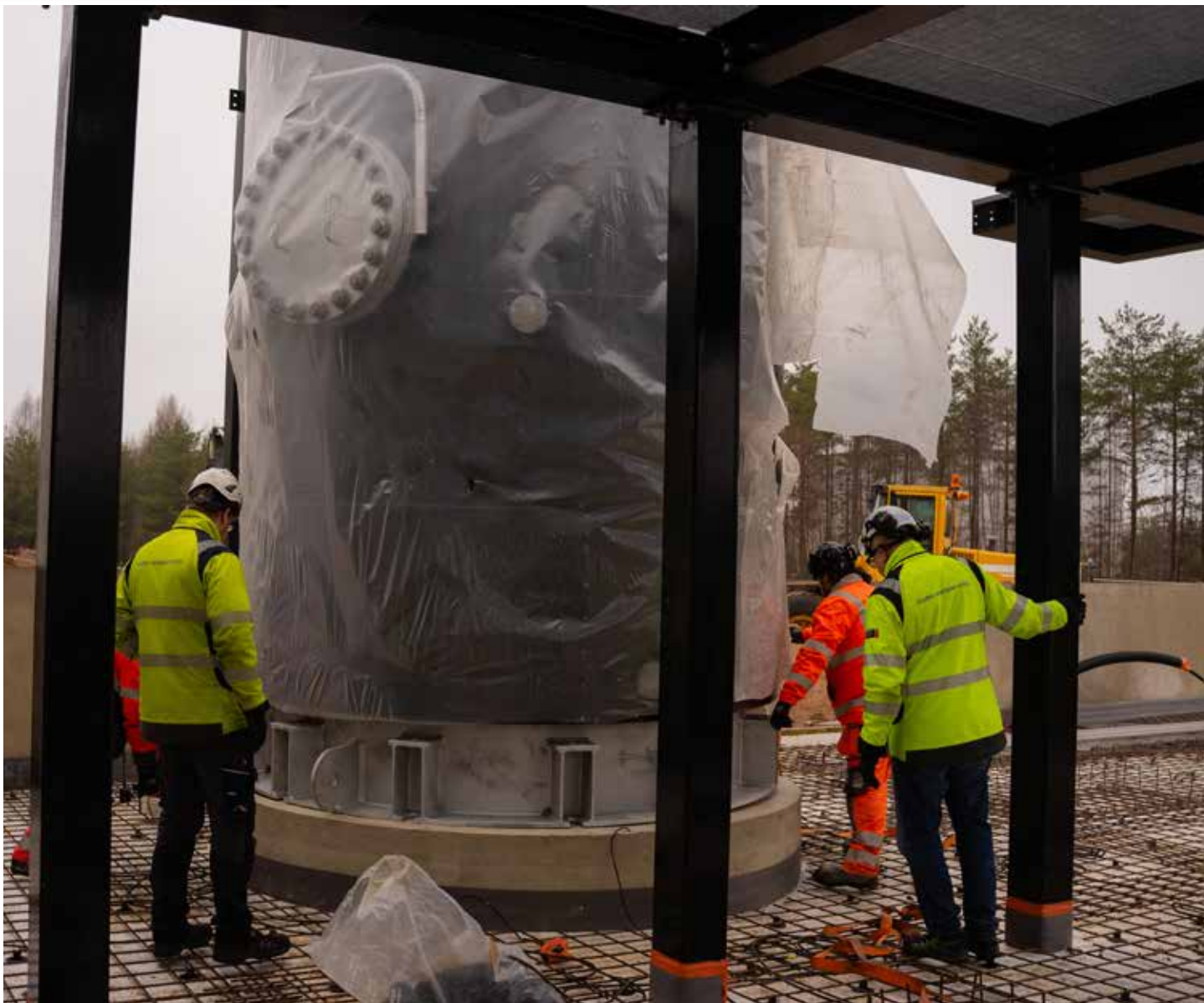
Electrode boilers are instrumental in generating revenue by absorbing excess power, enabling rapid, demand-responsive operation that aligns with market conditions.
