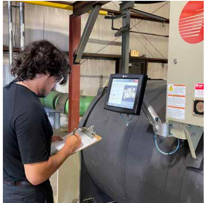
Trainee Brian Young works through various tasks to ensure operating parameters, like temperature, pressure and flow, are appropriate.
