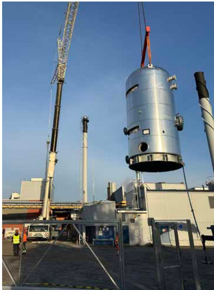
In the EU's broader decarbonization effort, high-voltage electrode boilers play a critical role in applications requiring rapid load absorption and grid stabilization.
