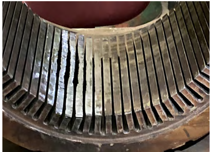
Damaged laminations will require proper repair to prevent rapid burnout of the motor after re-winding.
