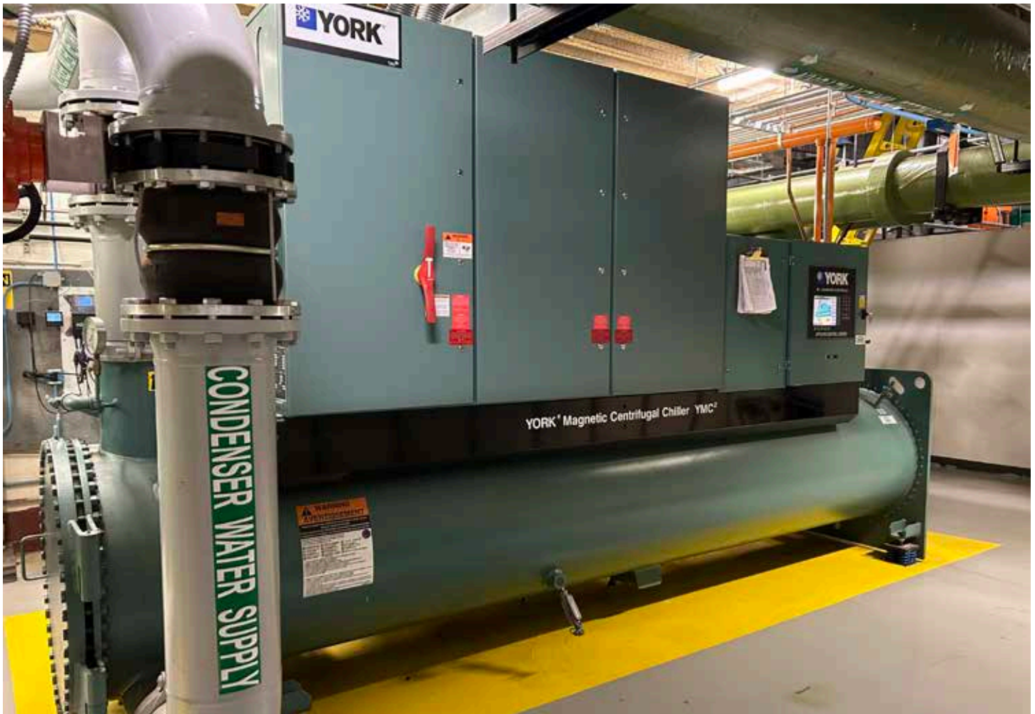
York centrifugal chiller.
