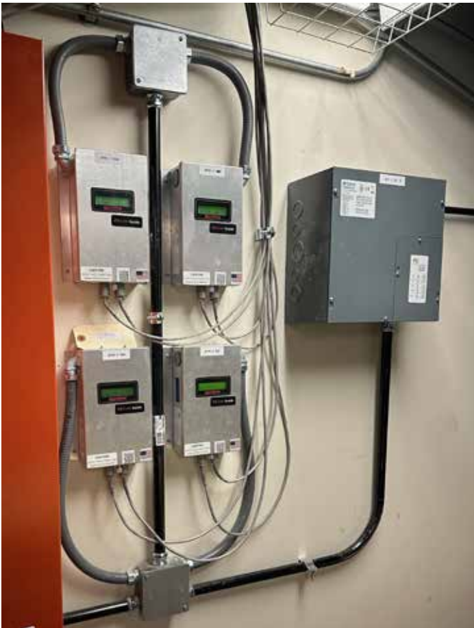
New airflow measuring stations on upgraded AC units for controlling new OA dampers.
