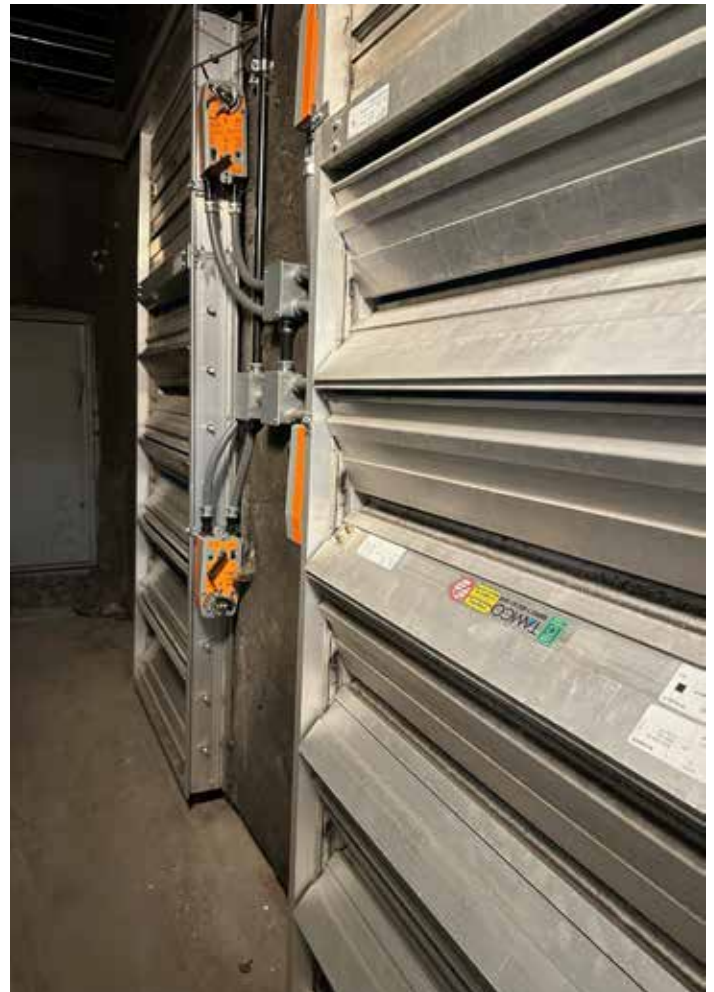
To enable air side economizing, new dampers were added to the existing AC units.
