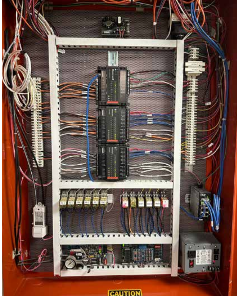
Updated controls, installed by AMS, for existing AC units
