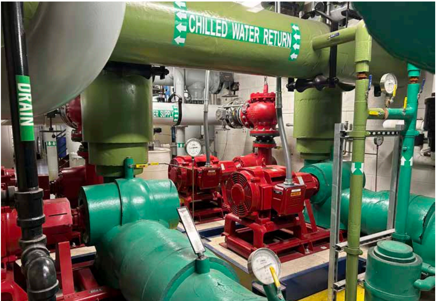
Chilled water system pumps.
