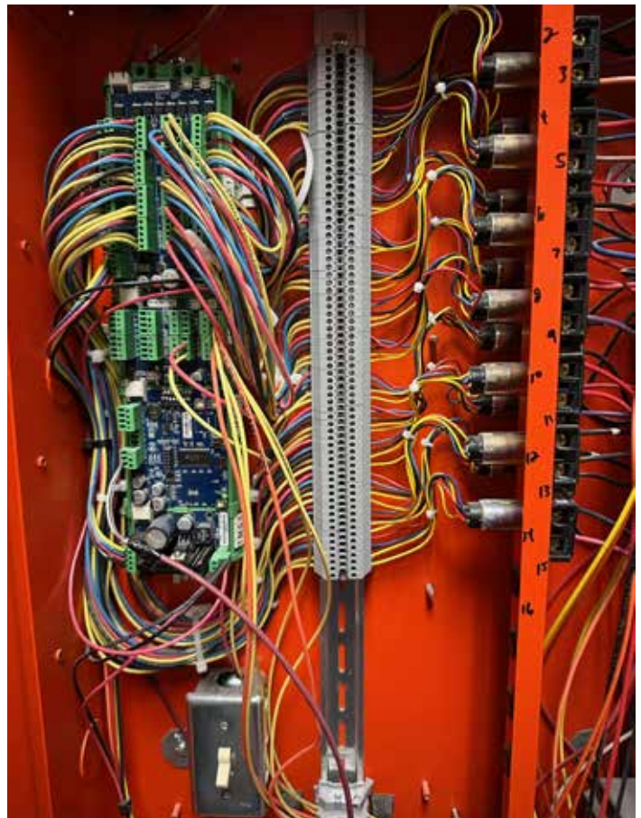
The current lighting panel, after retrofitting.
