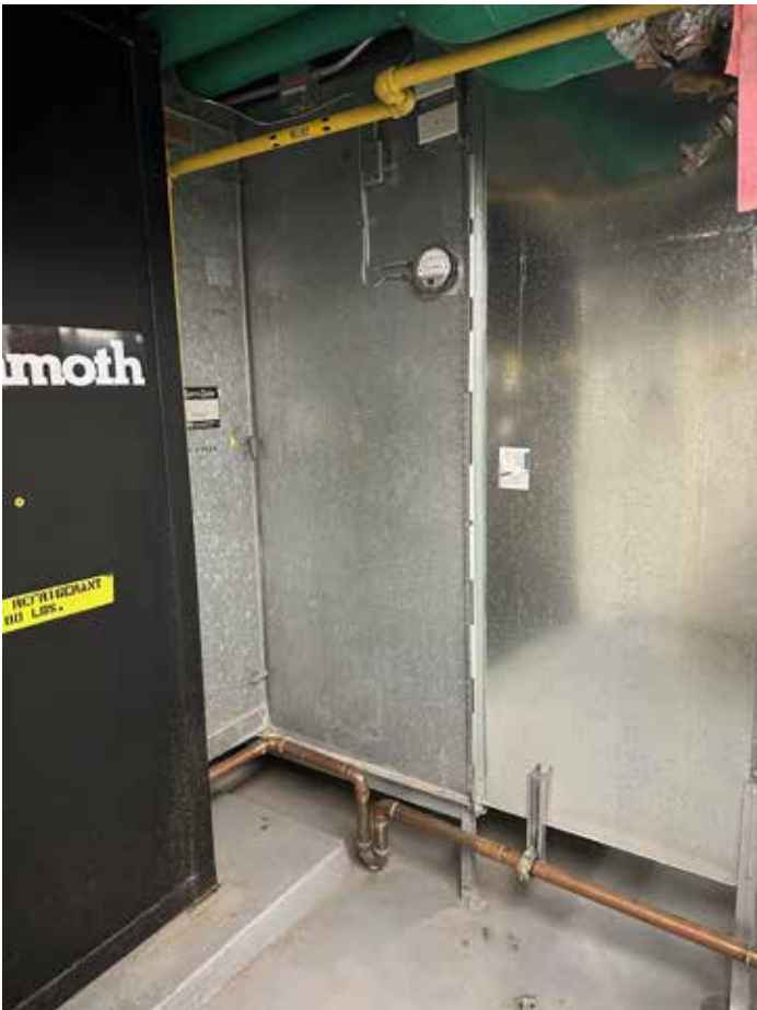
AMS added a new plenum to existing AC units in order to accommodate new OA dampers.
