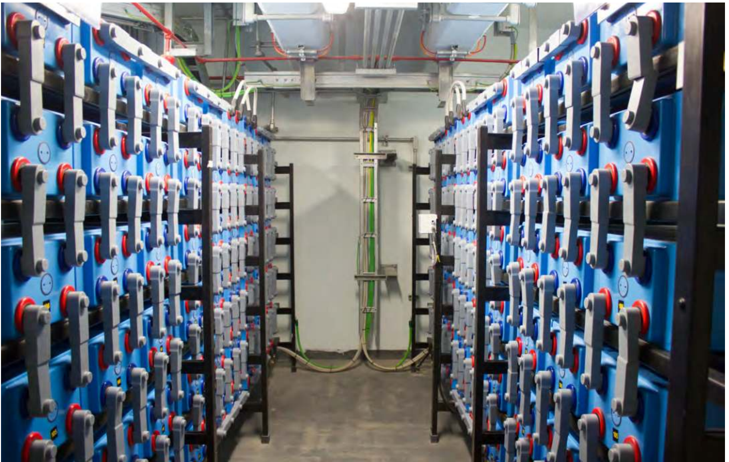
BESS are subject to thermal runaway conditions because, at their core, they utilize rechargeable batteries.
