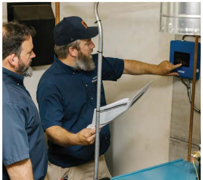
Two technicians set up the new smart boiler control.
