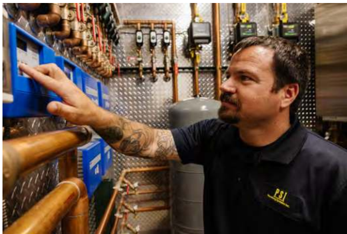
Brandon Content, at Plumbing Systems Inc., establishes a connection between several boilers and the tekmar control system that serves the large vacation home.
