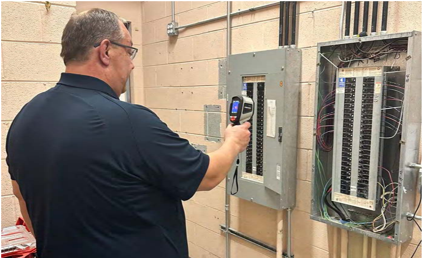
Bombard focuses on energy-efficient upgrades at CPS schools, like freon replacements, LED lighting and solar panel installs, heating system upgrades and adding electric vehicle charging stations.
