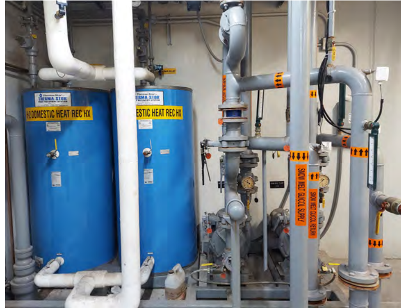
Domestic water heat reclamation exchangers.
