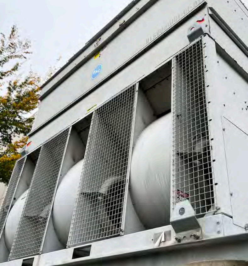
Baltimore Aircoil Company (BAC) cooling tower
