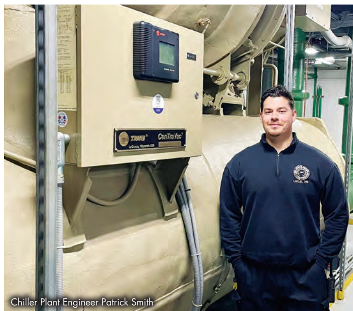
Chiller Plant Engineer Patrick Smith is responsible for oversight of the chemical treatment and daily readings.
