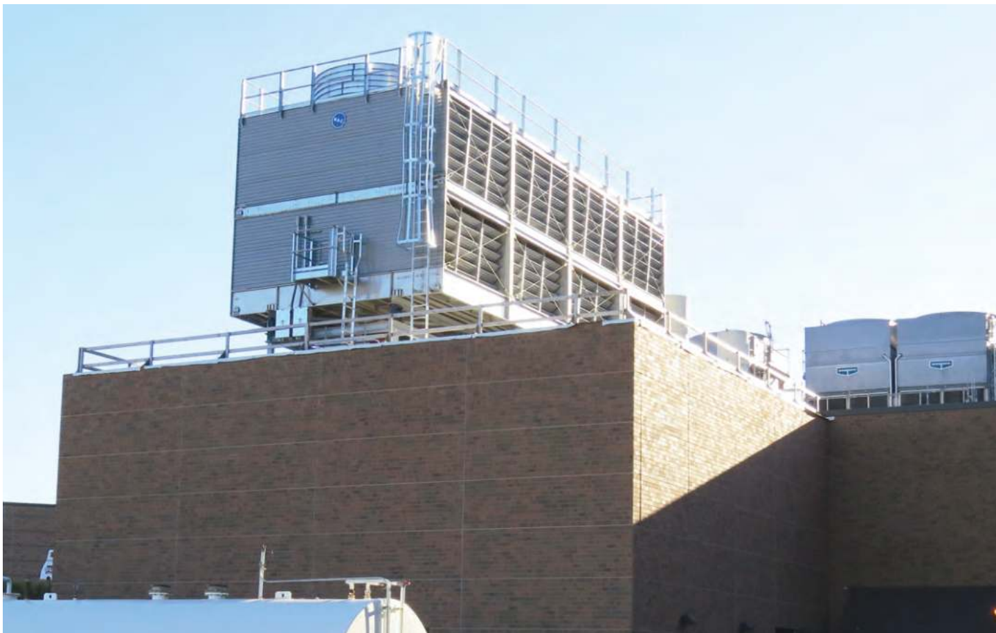
Your cooling tower and system need special care and attention below 45° F.
