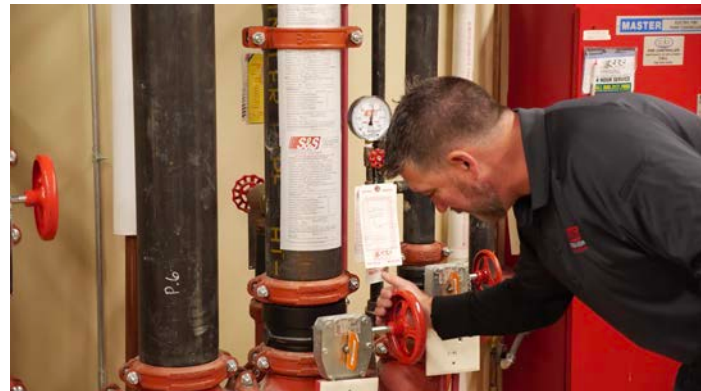
Verify that each fire sprinkler system in your community is inspected, tested, and maintained to ensure it will operate properly during a fire.
