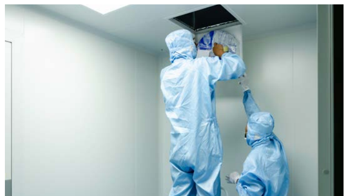
HEPA filters efficiently collect small particles and pathogens, but they do not deactivate live bacteria and viruses, making replacement potentially hazardous.
