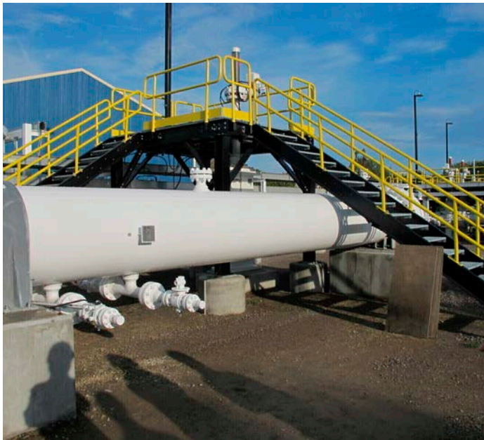
An above ground section of Enbridge's Line 5 at the Mackinaw City, Mich., pump station sits on Oct. 7, 2016. Attorneys for a Wisconsin Native American tribe argued Thursday, May 18, 2023, that a federal judge should order an energy company to shut down an oil pipeline the tribe says is at immediate risk of being exposed by erosion and rupturing on reservation land. U.S. District Judge William Conley indicated his reluctance to do so. (AP Photo/John Flesher, File)
