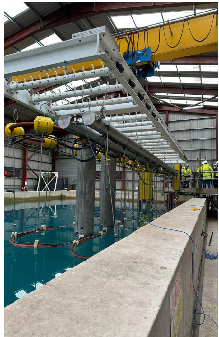
Forth's Deep Recovery Facility, which can hold 1.2 million litres of water, proved key in the sludge retrieval trials carried out by The Decommissioning Alliance.
