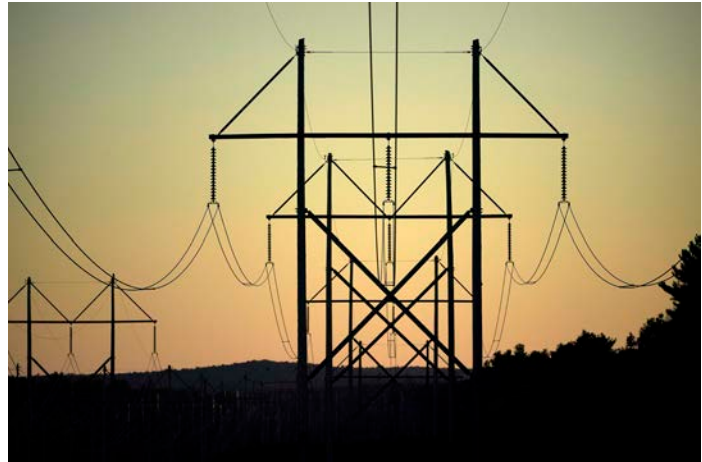
Central Maine Power utility lines are seen on Oct. 6, 2021, in Pownal, Maine. A Maine jury concluded on Thursday, April 20, that developers have a constitutional right to proceed with a $1 billion transmission project, despite being rebuked by state voters in a referendum. (AP Photo/Robert F. Bukaty, File)
