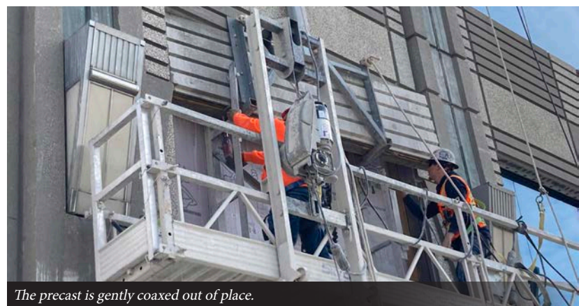
Once the precast is cut from the building and its weight transferred to the jack system, bolts are removed to free the brace from the side of the building, enabling the crane on the roof to begin lowering it to the ground.
